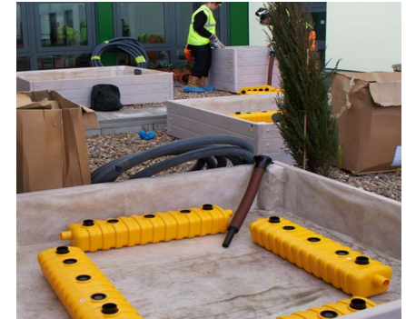
Water storage tanks and filler pipe
