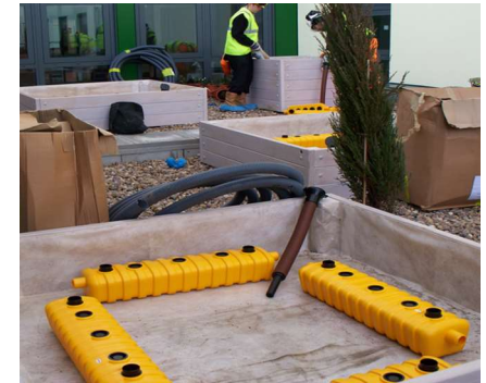
Water storage tanks and filler pipe
