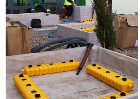
Water storage tanks and filler pipe
