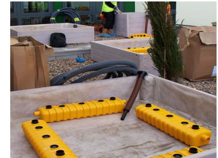
Water storage tanks and filler pipe
