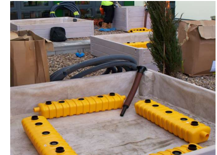
Water storage tanks and filler pipe
