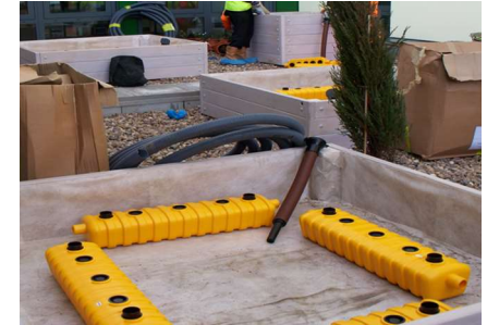
Water storage tanks and filler pipe
