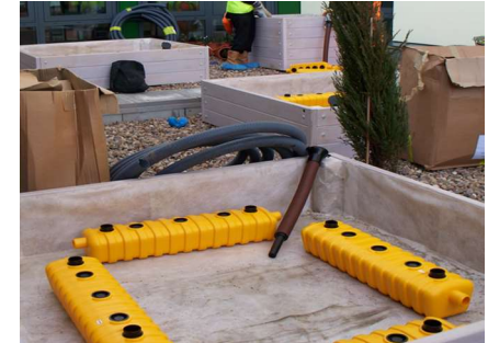
Water storage tanks and filler pipe
